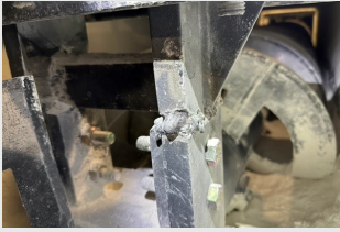
Existing Hanger Failed Due to Flexing and Fatigue
