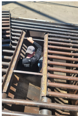
Very Limited Space for Floor Auger Created Need for KWS Engineered Solution
