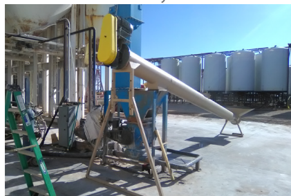
Screw Feeder is Completely Enclosed and Operation is Now Dust Free
