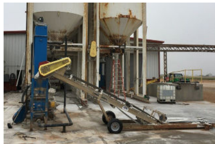
Mineral Powder is Offloaded from Live Bottom Trucks Using Belt Conveyor
