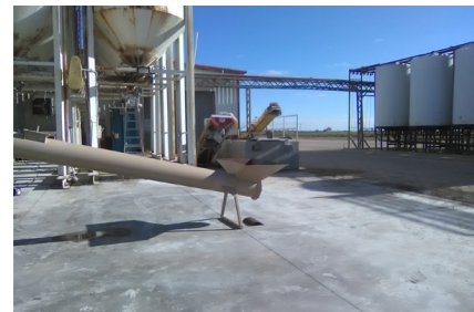
Live Bottom Trucks Discharge Materials to Hopper and Screw Feeder
