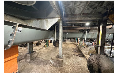
KWS Met Exact Specifications and System Fit Seamlessly into Existing Process
