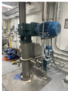
Drive End is Rigidly Supported to Eliminate Drive Movement
