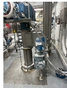
Vertical Screw Conveyor Housing is Supported at Floor Penetration
