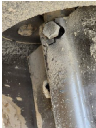
Repeated Stops and Starts Along with Improper Coupling Bolts Caused Screw Failure
