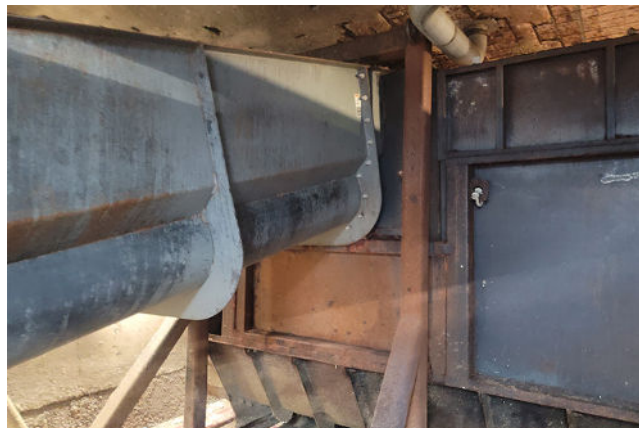
Key-Hole Trough Screw Conveyor is Coped to Fit to Surge Bin
