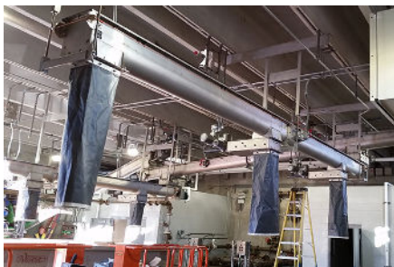
Screw Conveyors Can Be Reversed Only After Material Flow from Upstream Equipment is Completely Stopped
