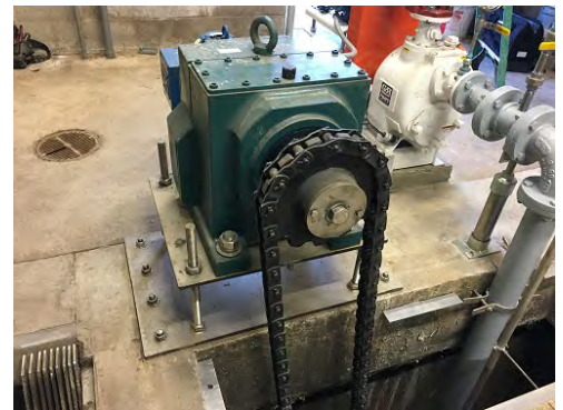
Motor and Gear Reducer are Located Above the Water Line
