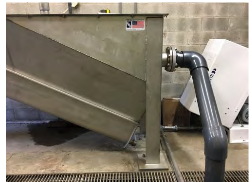
Clean Water is Returned to the Process
