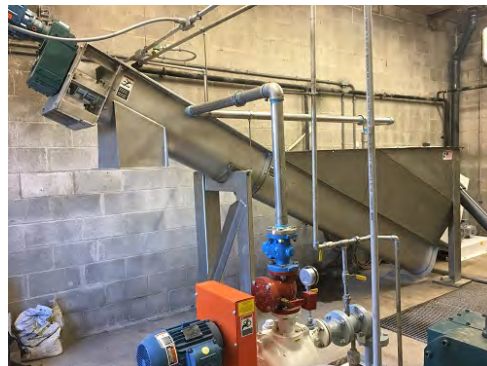
KWS Grit Classifier Separates Grit from Liquid
