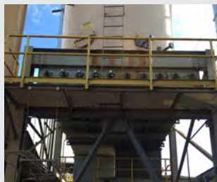
Existing Silo with 12-Screw Live Bottom Feeder
